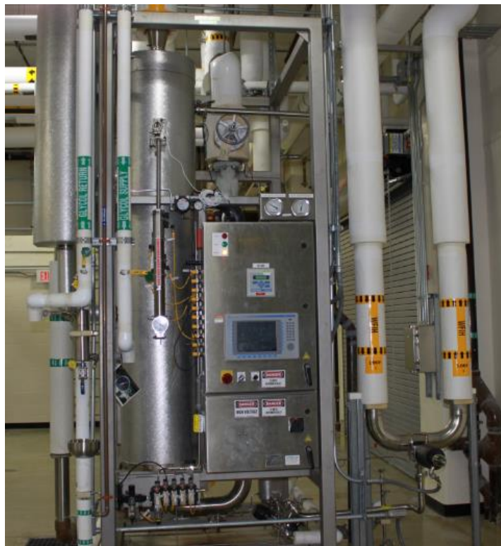
Figure 5-7. Steam generation system in a biomanufacturing facility
