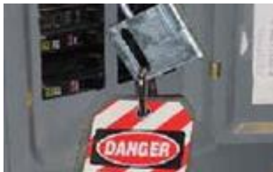
Figure 5-17. Example of a lock and tag on an energy source
