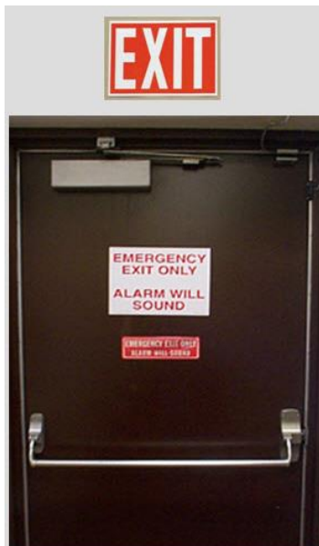
Figure 5-15. Clearly marked exit routes
